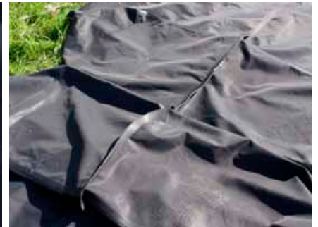
Make sure the weld on the bottom of the first SLAMDAM® follows the line of the next SLAMDAM®.
